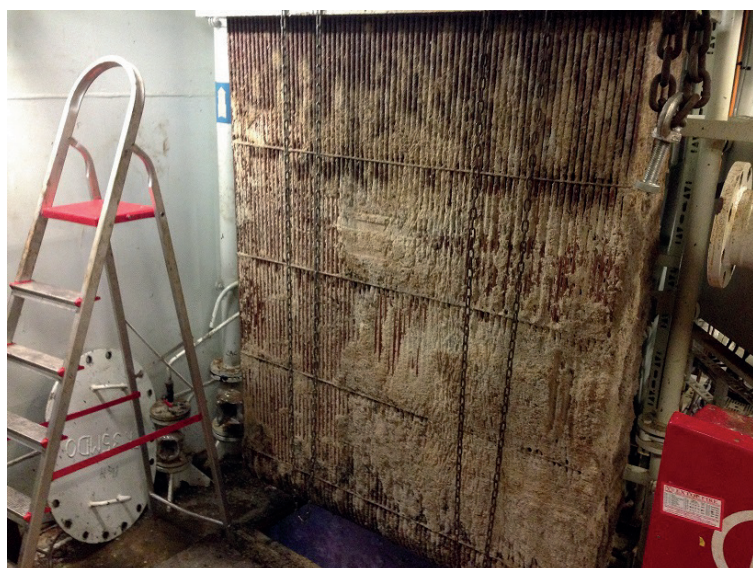
Building out a box cooler which is heavily contaminated with barnacles and mussels. Ready to take to our workshop for a proper chemical cleaning job.
